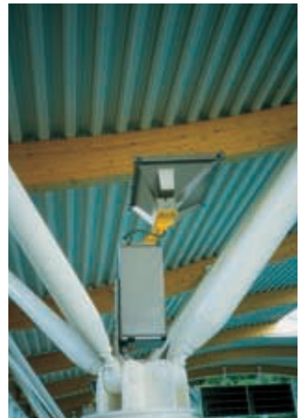
Detail of upward lights at the junction to the columns (photographer Derek Phillips).
