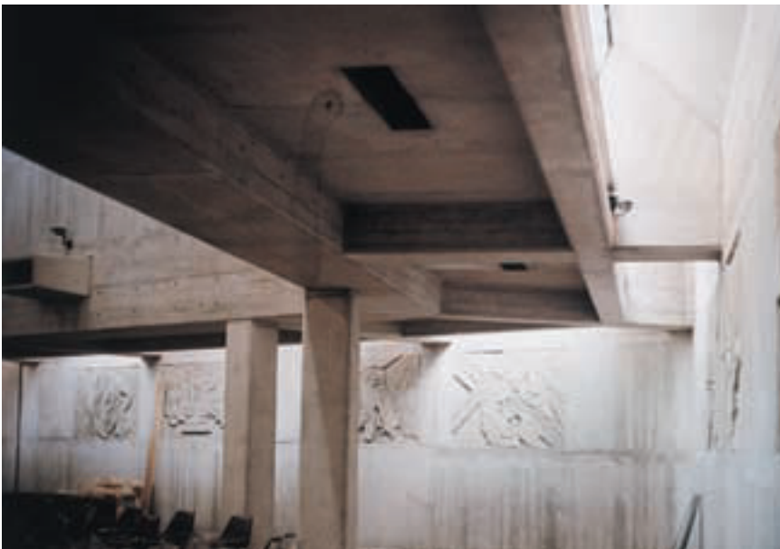
Ceiling detail allowing the entry of both daylight and artificial light (Photographer Derek Phillips).
